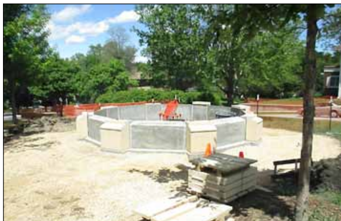
Ground pool base construction of the new "Boy in Blue" Blue Earth County Civil War Memorial in Lincoln Park, Sept. 2013.
