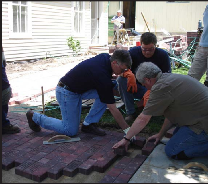
Hometime crew laying the new paver walk. L - R: (kneeling in front ) Chris Balamut and Dean Johnson.
