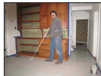
Doug Laven putting the final coat of paint on the kitchen floor.
