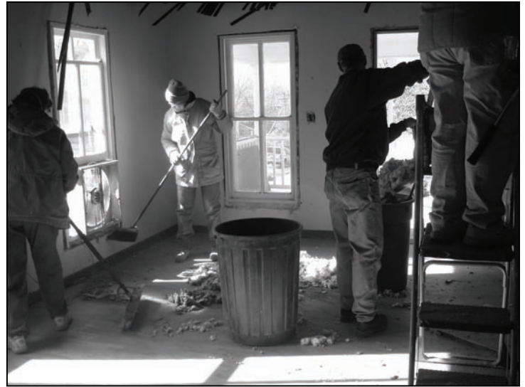
Volunteers working in the dining room. Cleaning up the old plaster and insulation was a big job. We filled many dumpsters (provided by Goodrich Construction) with debris that was hauled to the landfill. October 24, 2006
