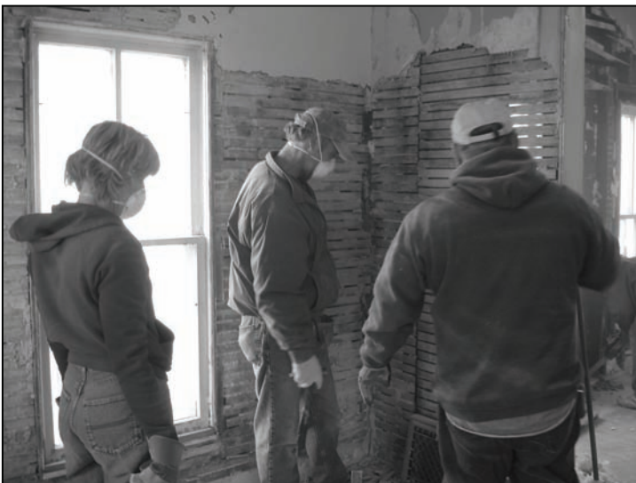
(L-R) Patti Sjulstad, Denny Weis and Judd Nelson in the front parlor during demolition. The old plaster and insulation was removed from all the walls.
