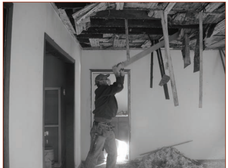
Denny Weis working on the dining room ceiling. The dining room and kitchen ceiling had many layers of old newspapers below the insulation. The newspapers were dated late 1930s and early 1940s.
