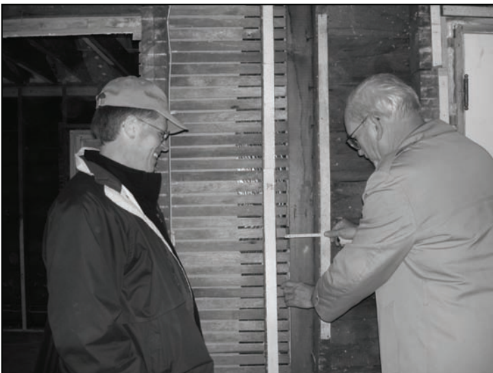
(L-R) Chris Balamut and Tom Hagen looking for clues to original construction.
