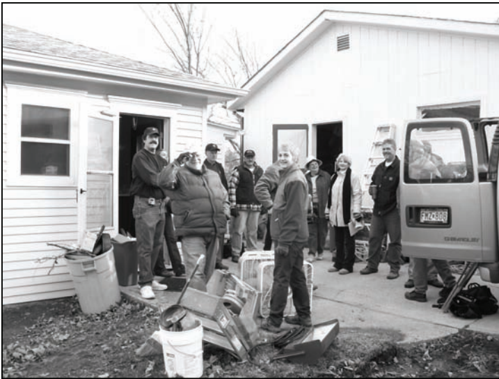
Hometown returns to work and film interior restoration at Betsy's house. October 24, 2006.
