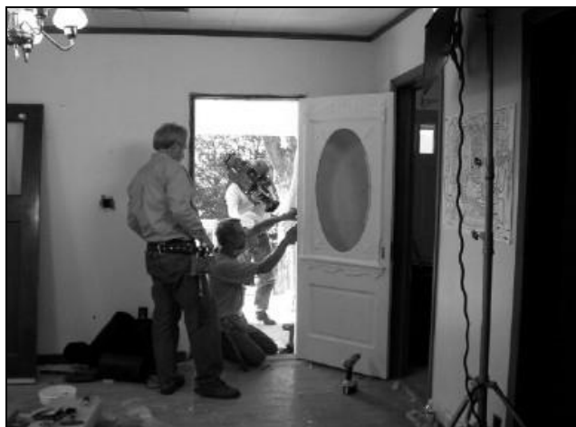
Installing the new front door. L to R: Dean Johnson, Dennis Weis and in the background is videographer, Jeff Lyman.
